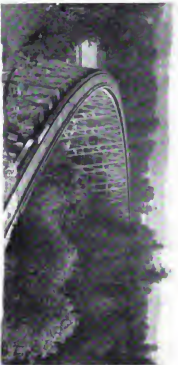
A RAILROAD BRIDGE IN ELNRUN TOWNSHIP (1,000 feet long, 100 feet high, all built on a curve.)
